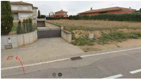
HIDRANT 2 CARRER TEMPLE
